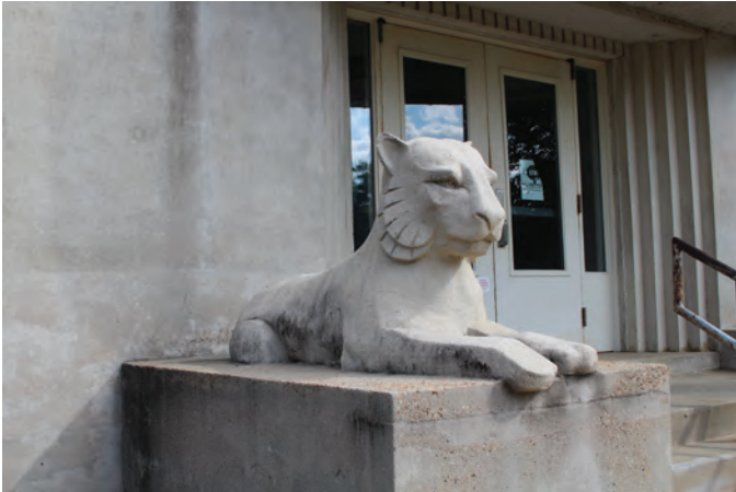
Fig. 4: Exposed concrete surfaces and sculpture at the Bailey Magnet School, Jackson, Mississippi
