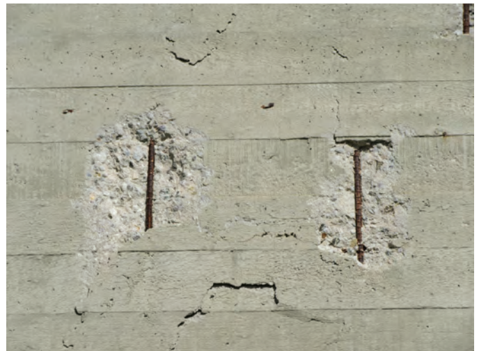
Fig. 9: Delamination and spalling at exposed concrete are examples of distress and deterioration that should be documented as part of a visual condition survey
