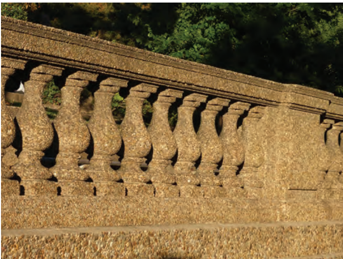
Fig. 5: Exposed aggregate at a historic concrete balustrade
