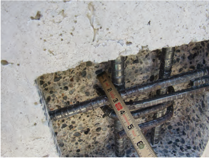
Fig. 10: Removal of concrete beyond the corroding reinforcement bar to allow for removal of corrosion product and to address the underlying distress mechanism
