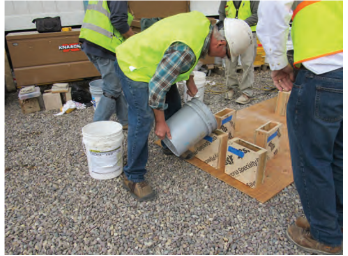
Fig. 11: Completion of off-building trial samples and mock-ups prior to the start of repairs to confirm appropriate performance of the concrete mix design, placement procedures, and finishing techniques
