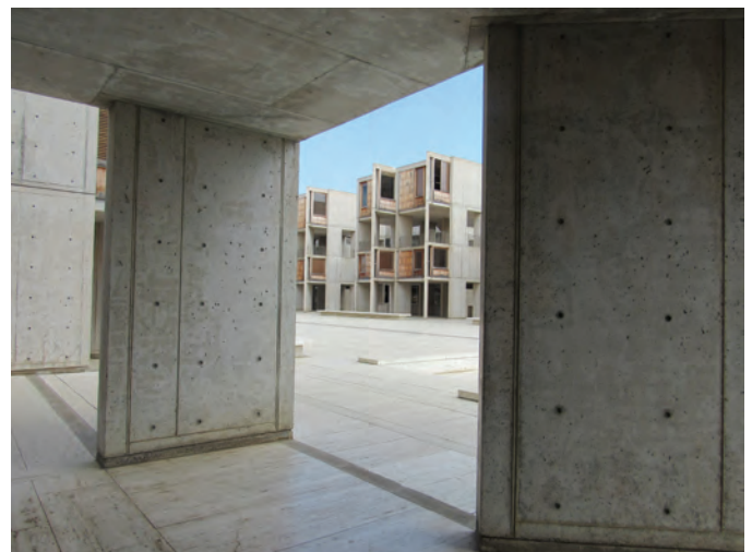
Fig. 3: Exposed concrete finish at the Salk Institute for Biological Studies in La Jolla, California, designed by Louis Kahn
