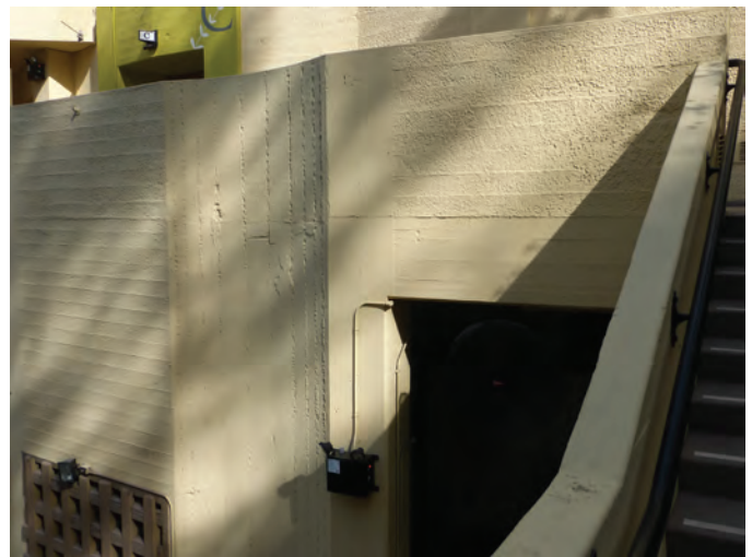
Fig. 8: Due to variations in formwork and finishing techniques, there are visible differences in texture, even after a coating has been applied
