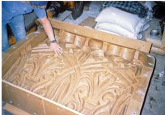
Intricate multi-piece fiberglass and rubber molds provided for accurate and efficient repair of the highly sculpted ornamental concrete components
