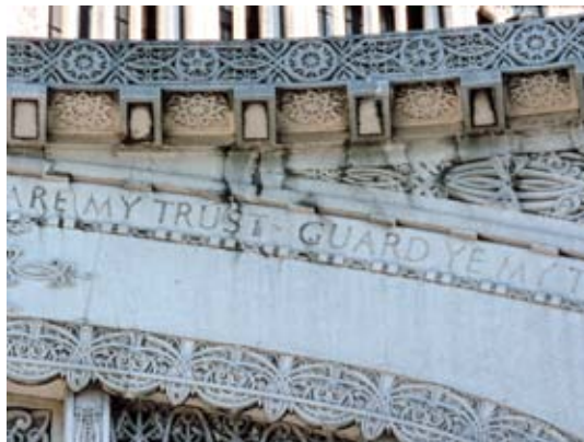
Before the cleaning began in 1989, the temple was covered with black crusts of gypsum crystals, organic growths, and extensive stains of atmospheric pollution
